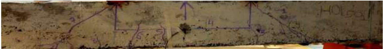
Fig.11: Crack Pattern of Hollow (50mm) beam
