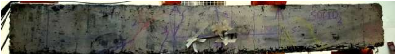
Fig.9:Crack Pattern of Solid Beam`
